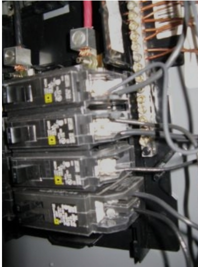
Double tap breaker in remote panel. Recommend repair.
