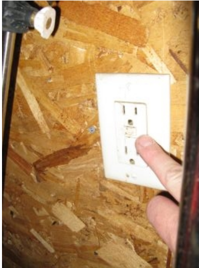
Outlet not working at time of inspection.
