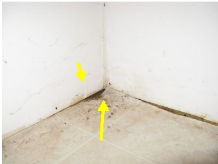
Moisture was noted at time of inspection in basement bathroom closet corner.
