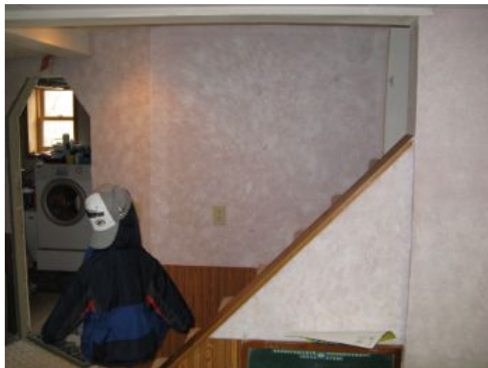
Open side of stairway. Recommend railing and or/ balusters.
