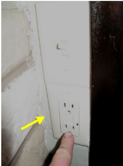
Outlet was found to be possibly wired wrong.
