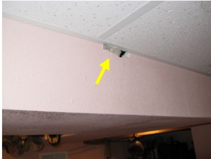
Possible asbestos noted at time of inspection.
