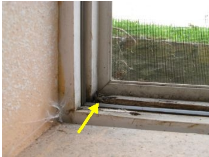
Basement bedroom window. Wood damaged in this area. Recommend repair to gain weather tight seal.
