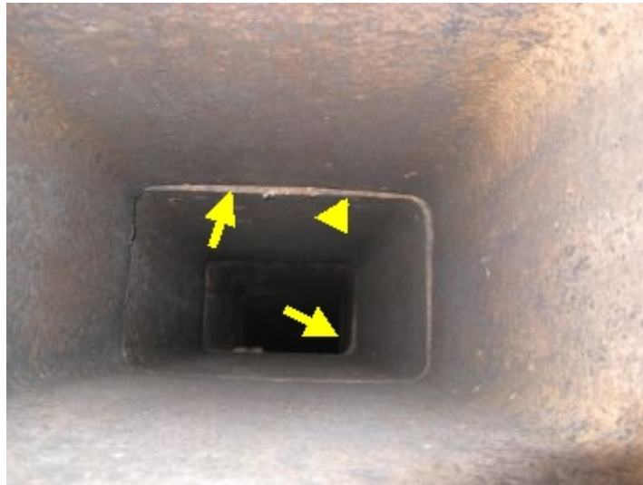
Appeared to be a gap or misalignment.
