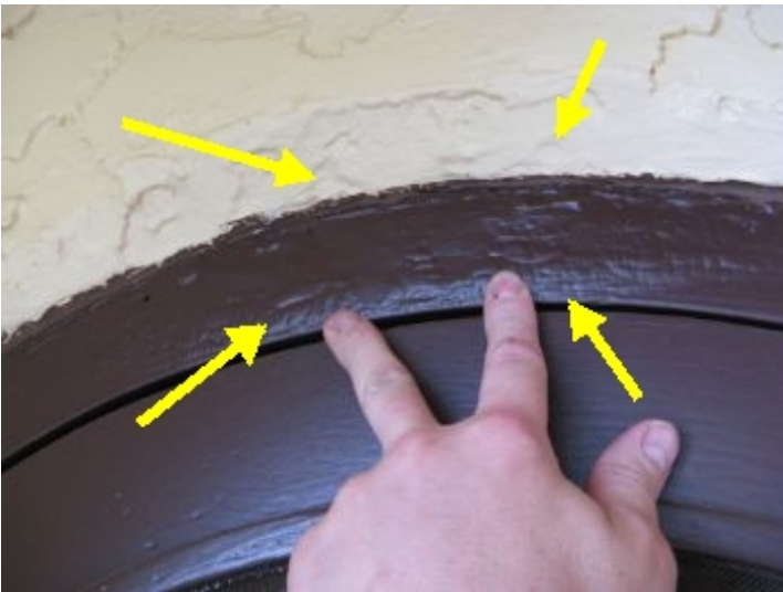
Bubbled paint over front entry door.
